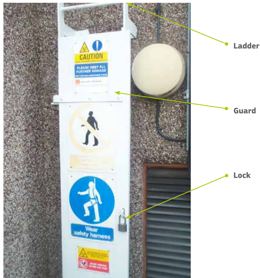
Figure 9.2 — Use of ladder guard to restrict access to strong fields on a rooftop
