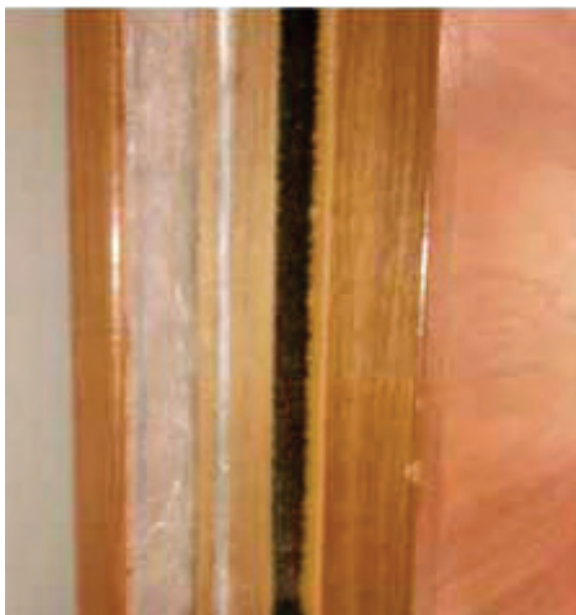
Figure 14: Side view of the scan room door. Lead lining approximately 4 mm wide can be seen and provides additional shielding
